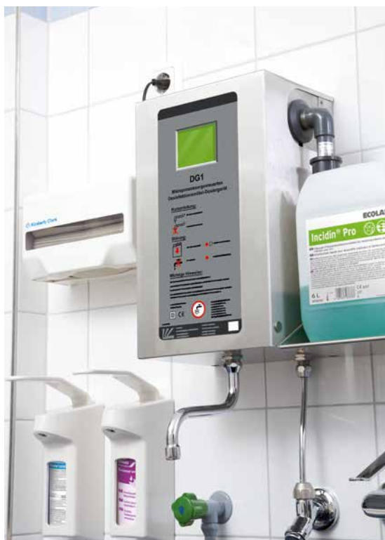
Fig. 1: Decentralised dosing device
