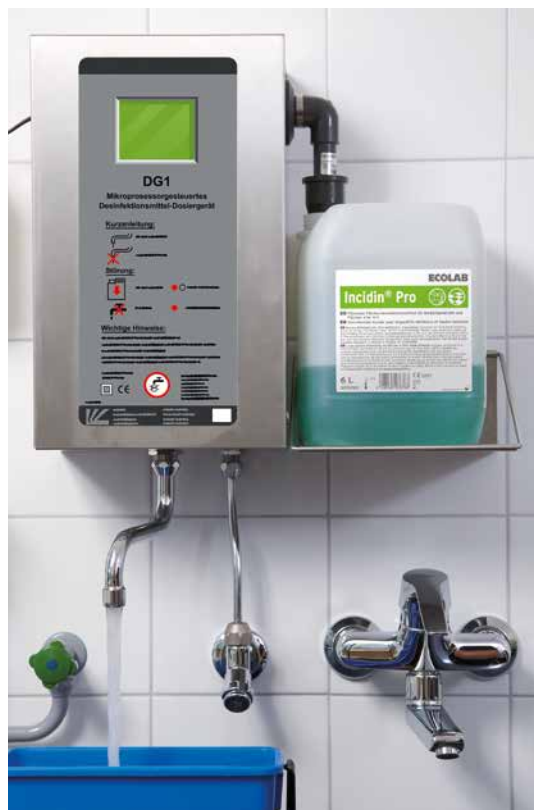
Fig. 2: Decentralized dosing device
